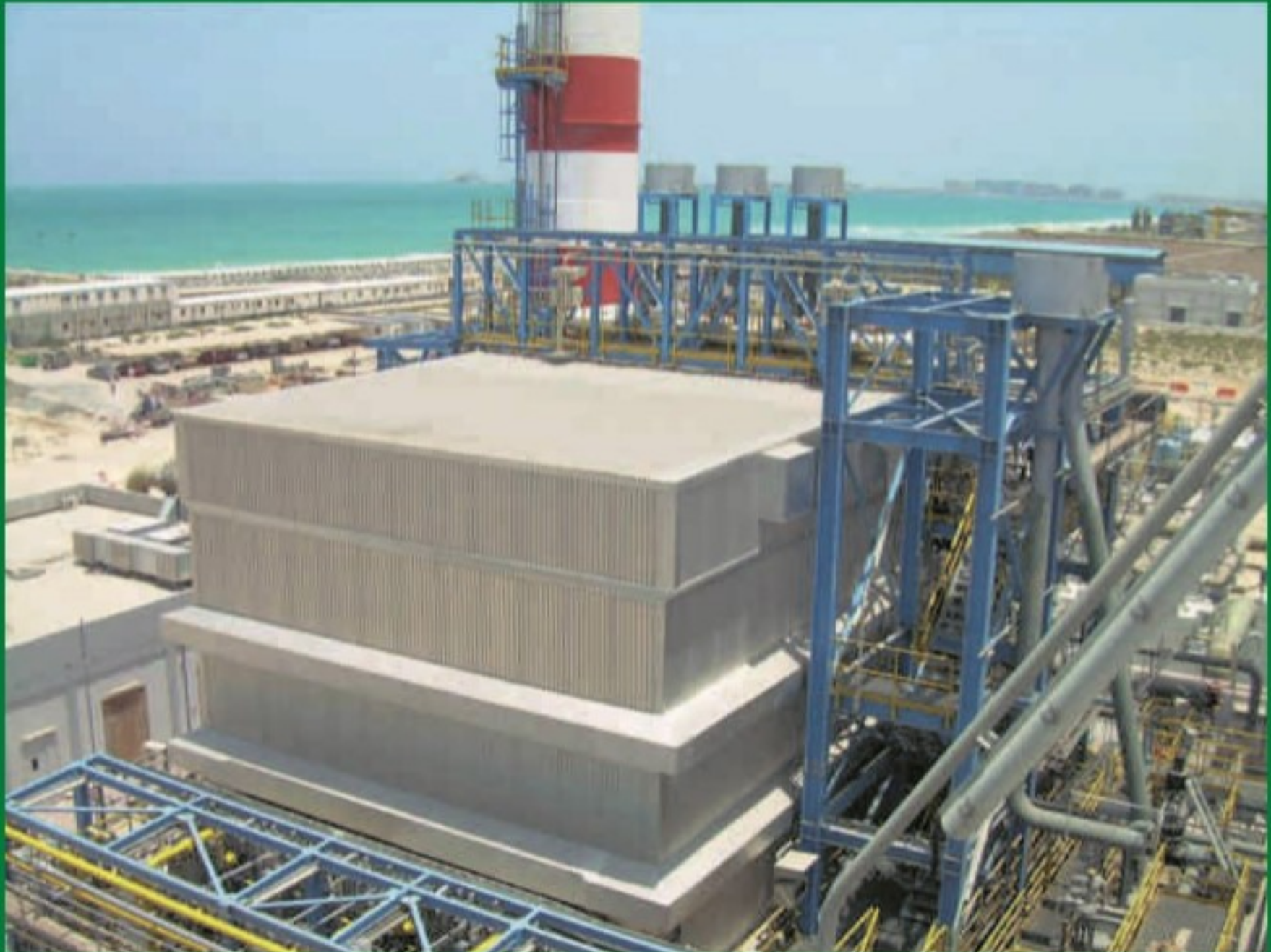
Jebel Ali Power Plant - UAE
