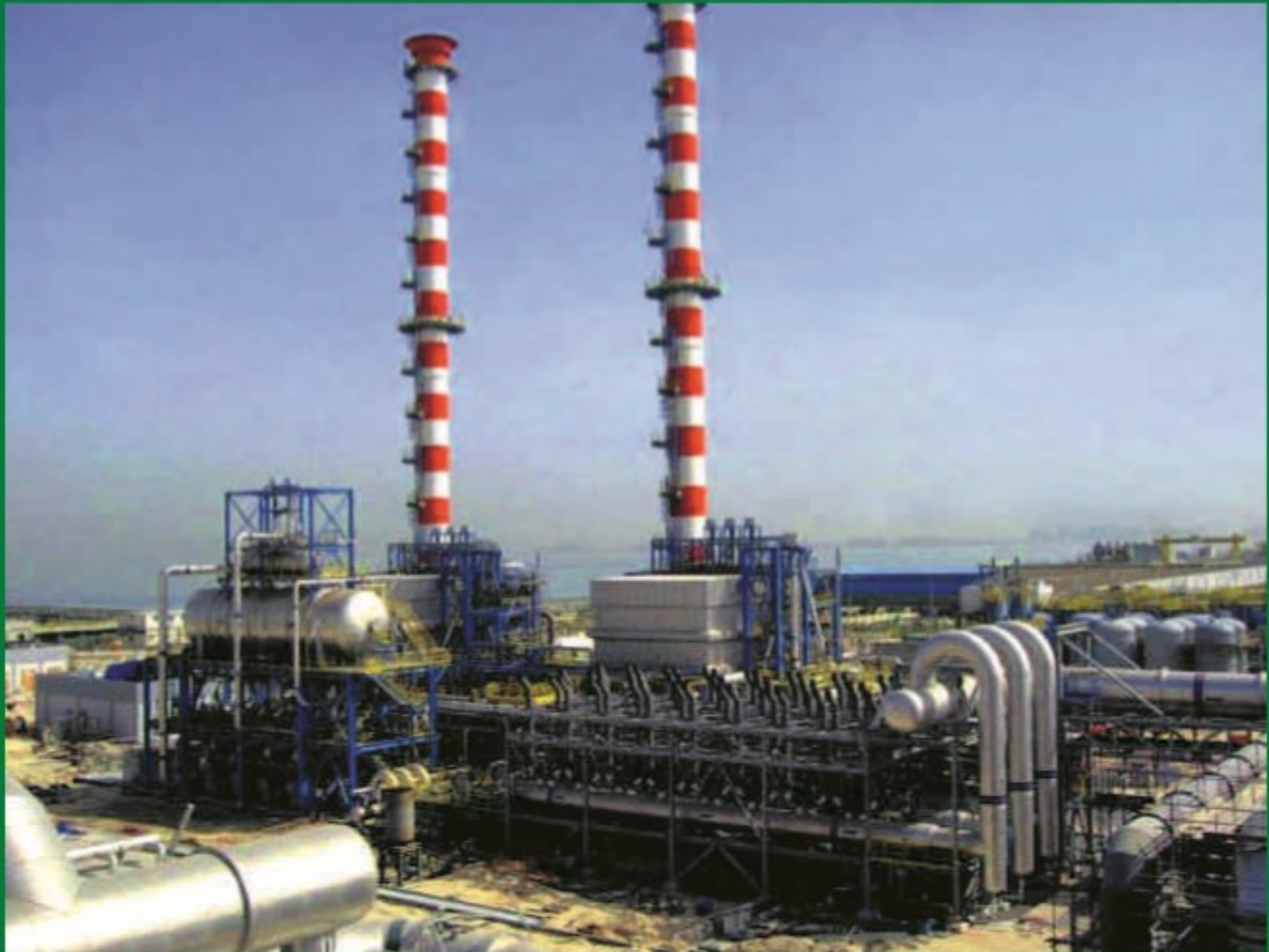
Jebel Ali Power Plant - UAE
