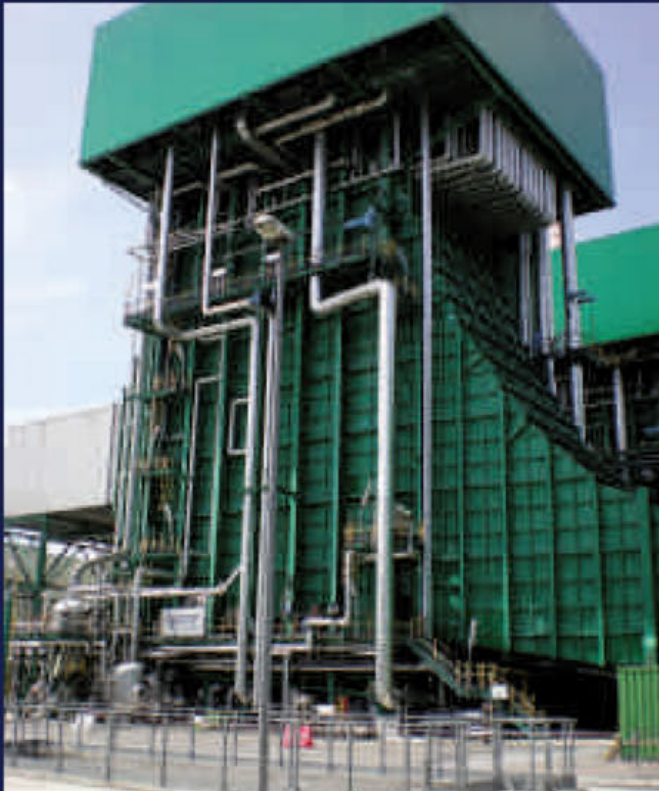
Tavazzano Power Plant - Italy
