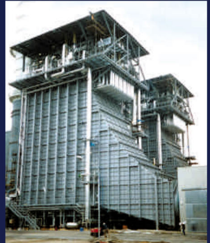
Piacenza Power Plant - Italy
