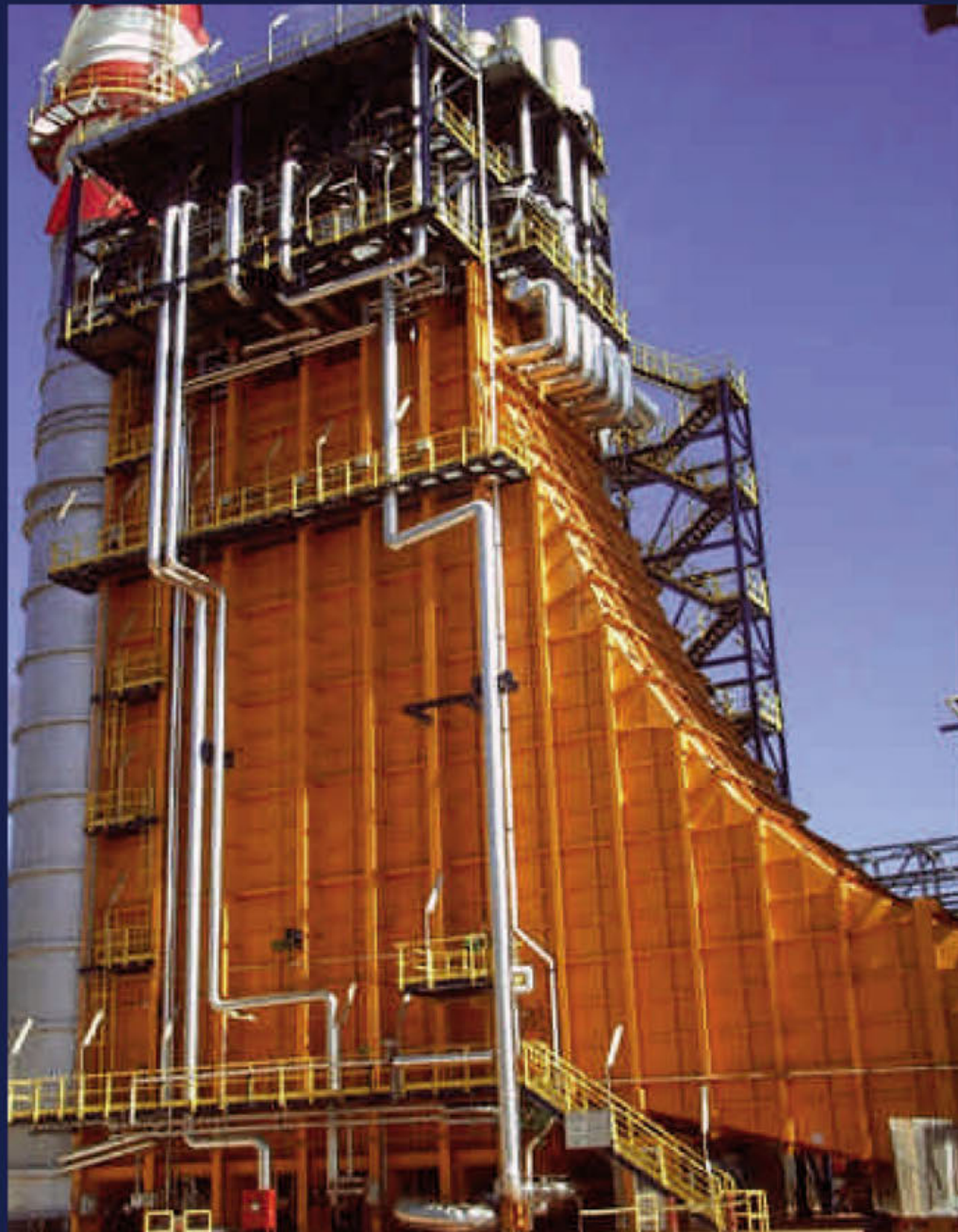
Ibiritè Power Plant - Brazil
