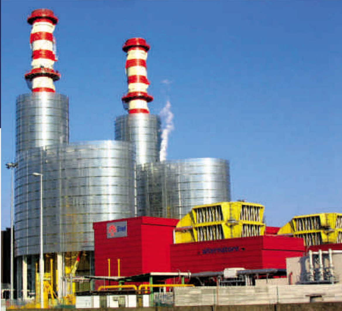
Porto Corsini Power Plant - Italy
